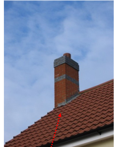
Modern chimney, 'signed off' by Building Control and warranty provider — in the wrong place
